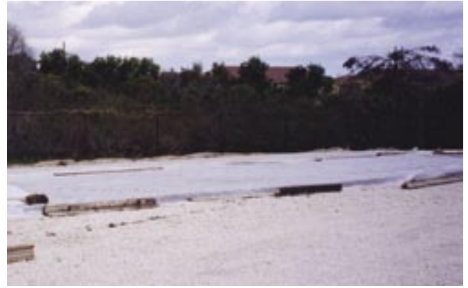
Fig. 7: Plastic sheeting is typically used to retain moisture in the pavement mass for curing
