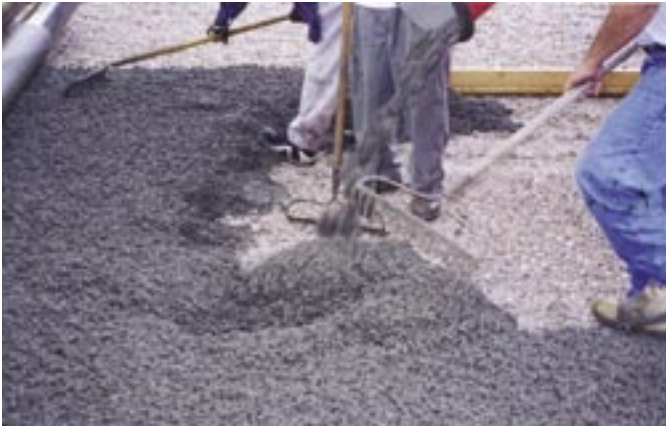
Fig. 2: Concrete should be raked to an approximate elevation as it leaves the truck
