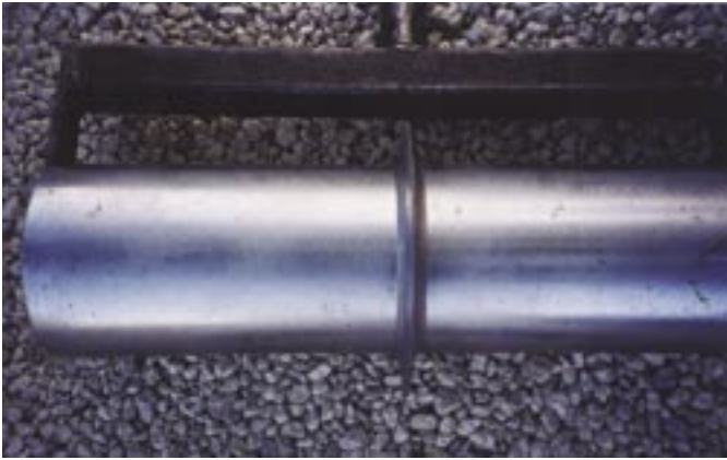
Fig. 6: A rolling/jointing tool may be used on pervious concrete, rather than saw cutting
