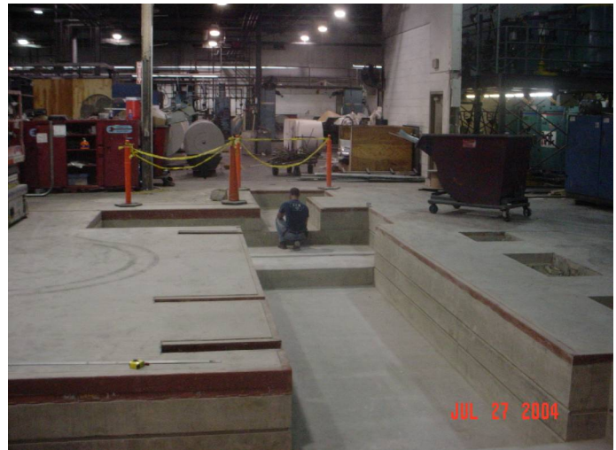
Prepping the finished printing press foundation pad for the heavy press equipment that will be placed within days of the finished pour. This project had five day breaks of 5700 psi., allowing the customer to stay on schedule.
