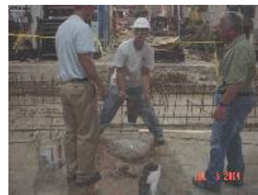
Measuring the "spread" (22-24") of the SCC. Notice the upside down slump cone.
